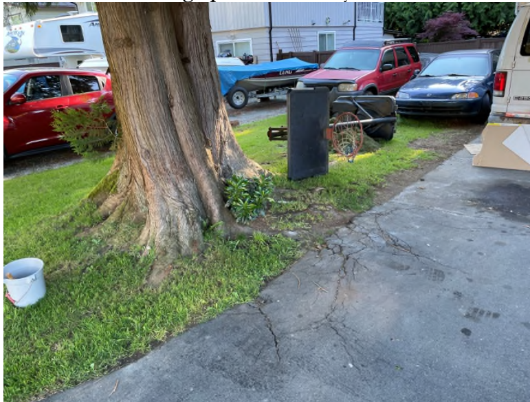
Photograph 2: Tree #63 offsite with roots lifting asphalt.
