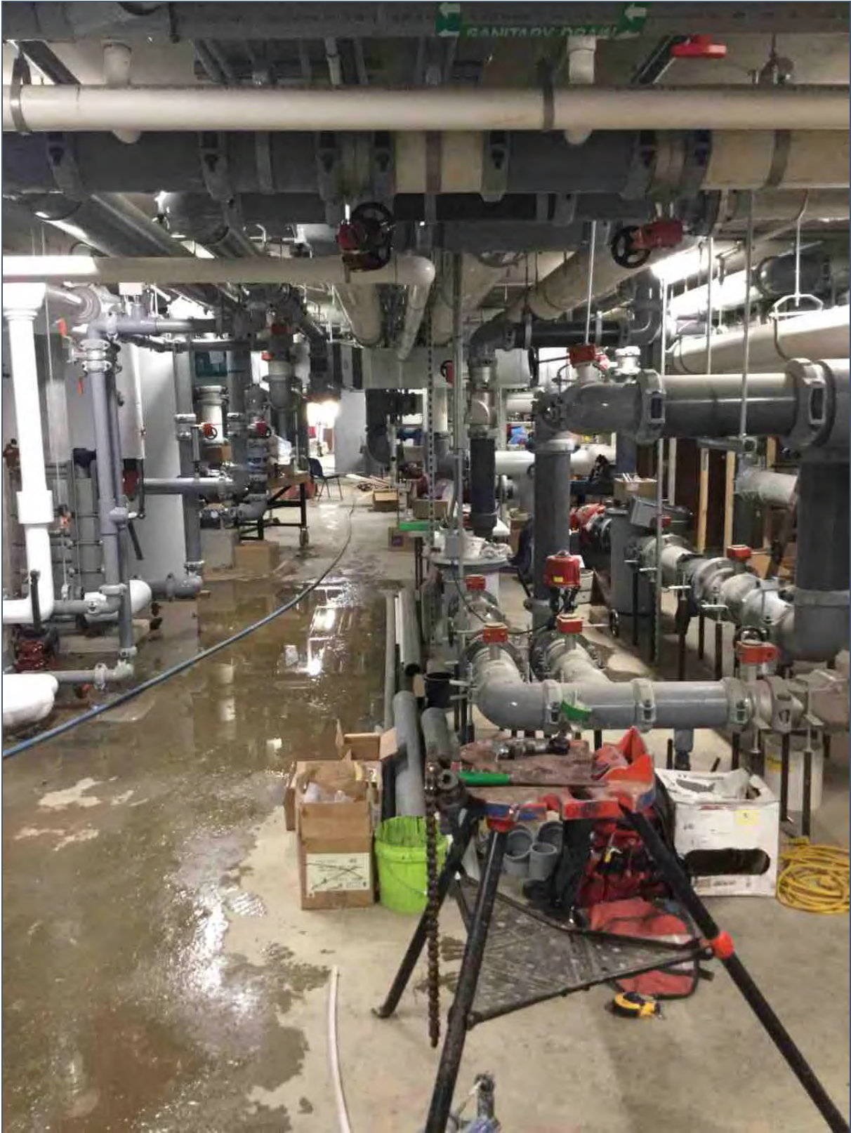
Phase 1C – Pool equipment room
