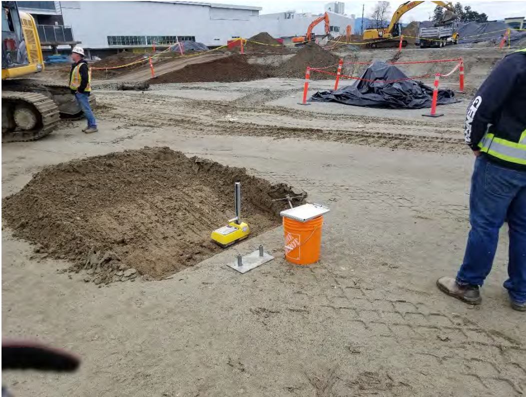
Photo 1 – Compaction testing of fill placed on November 14, 2019 (Item 3). [photo taken by JAL and dated 20191118]
