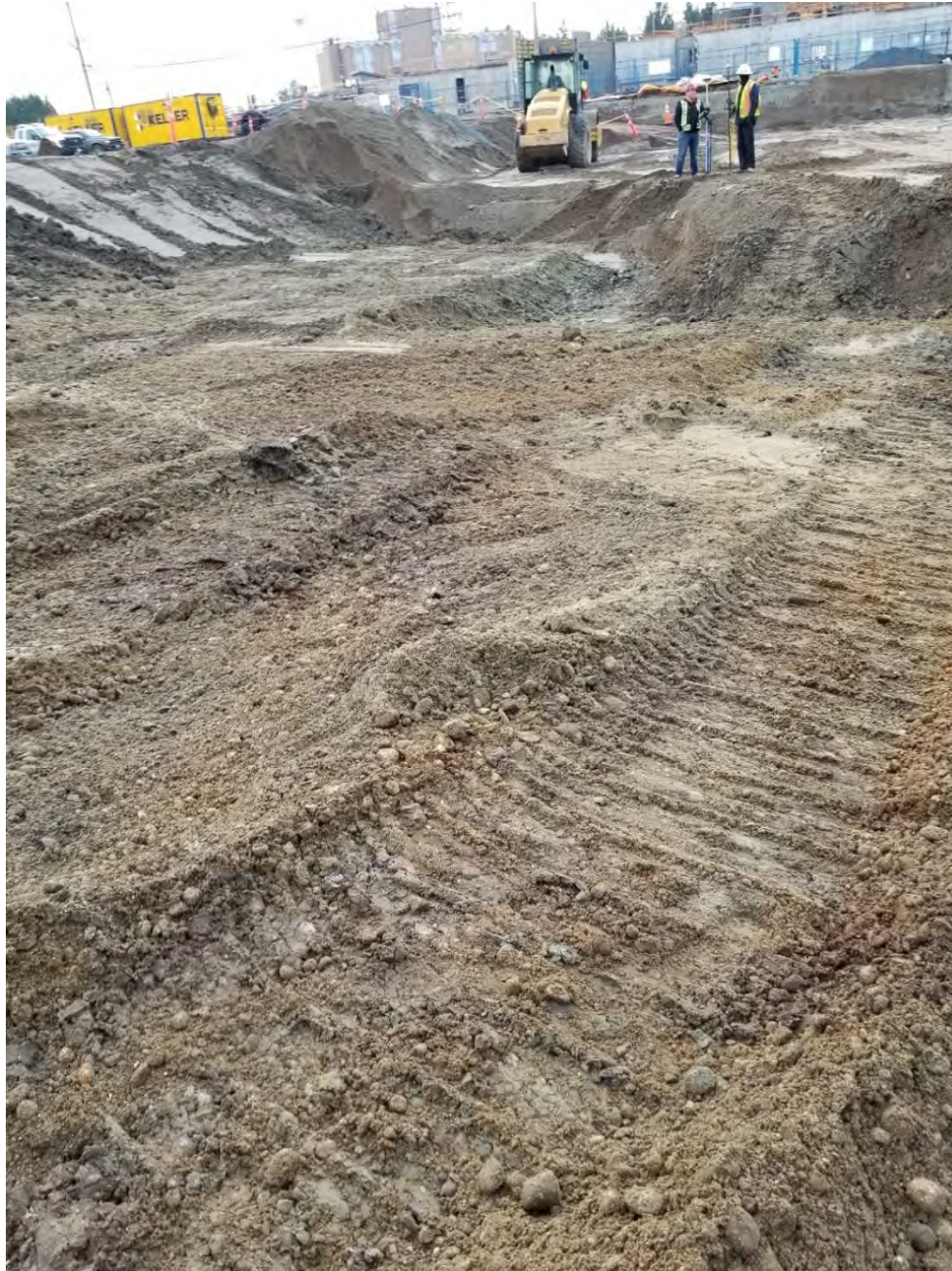
Photo 1 – Looking south. Approved subgrade area (Item 3). [photo taken by JAL and dated 20191114]
