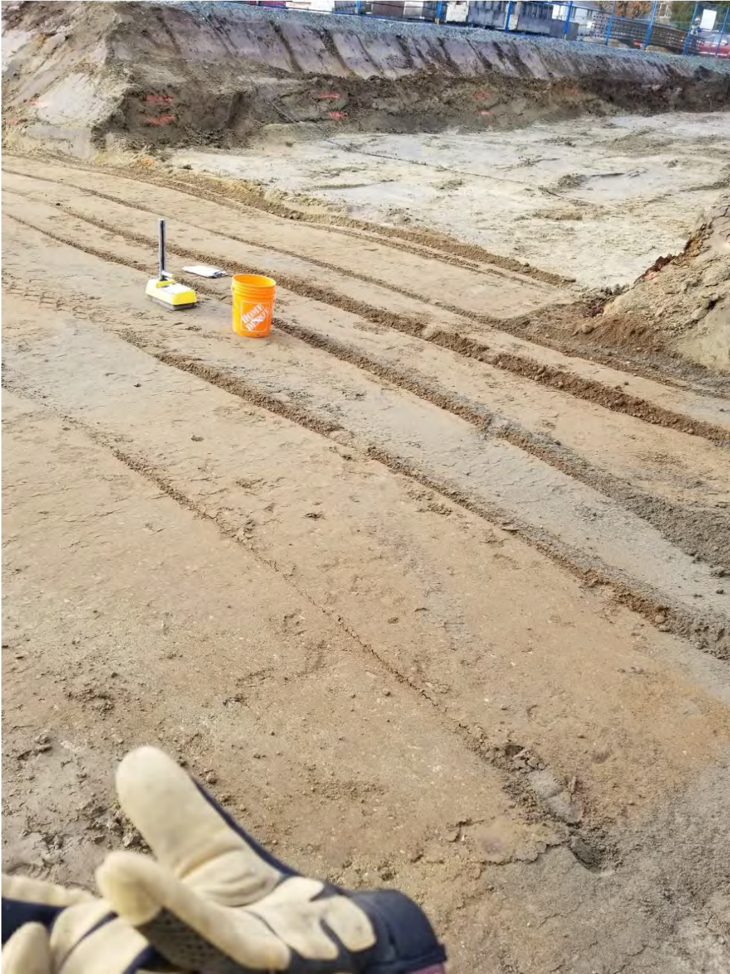
Photo 2 – A lift of Sand and Gravel placed over the west portion of the approved subgrade area. The lift varied in thickness to level out the sloping subgrade (Item 5). [photo taken by JAL and dated 20191114]
