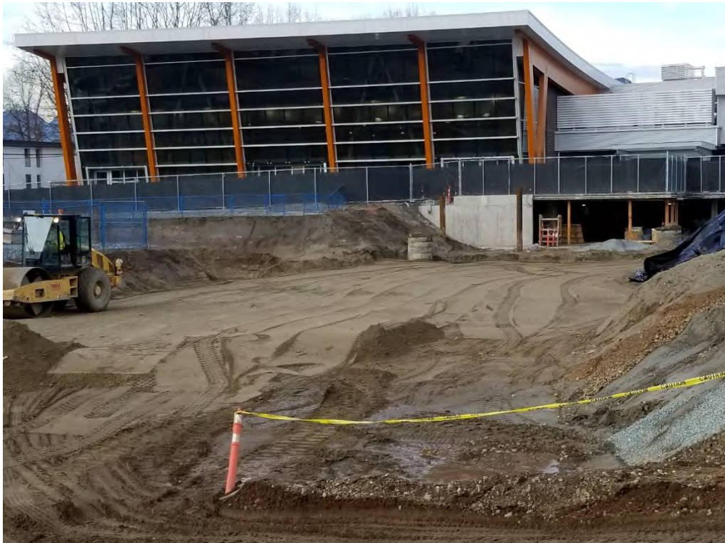
Photo 4 – During compaction of the last lift of fill (Item 9). The lift extended from the north of the excavation up to the well point near the southwest edge of the of the excavation. [photo taken by JAL and dated 20191114]
