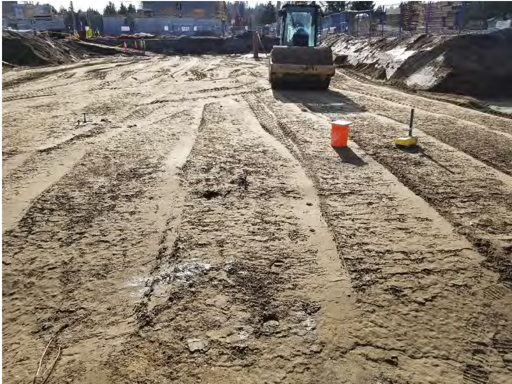
Photo 3 – Second lift placed across the approved subgrade area (Item 6). The base of the entire is now flat (Item 7). [photo taken by JAL and dated 20191114]
