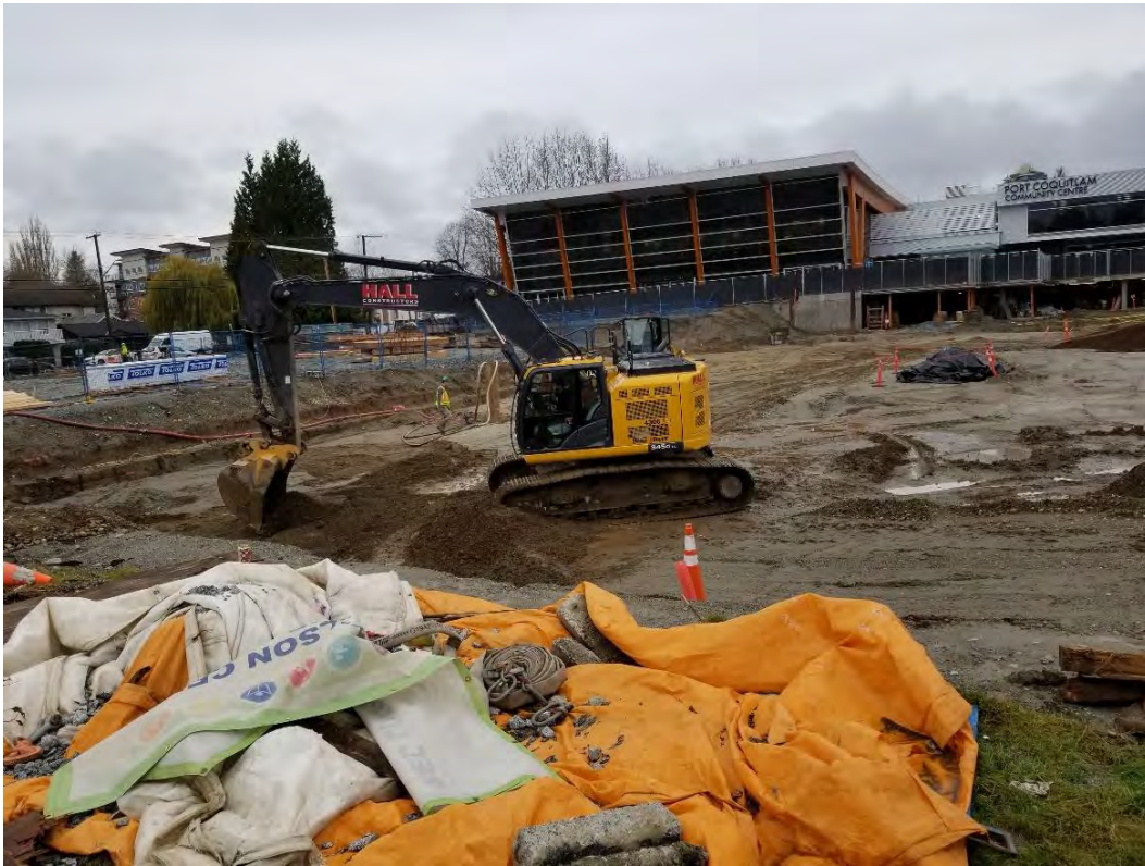
Photo 2 – Removal of standing water and saturated material along south end of excavation (Item 4). [photo taken by JAL and dated 20191118]
