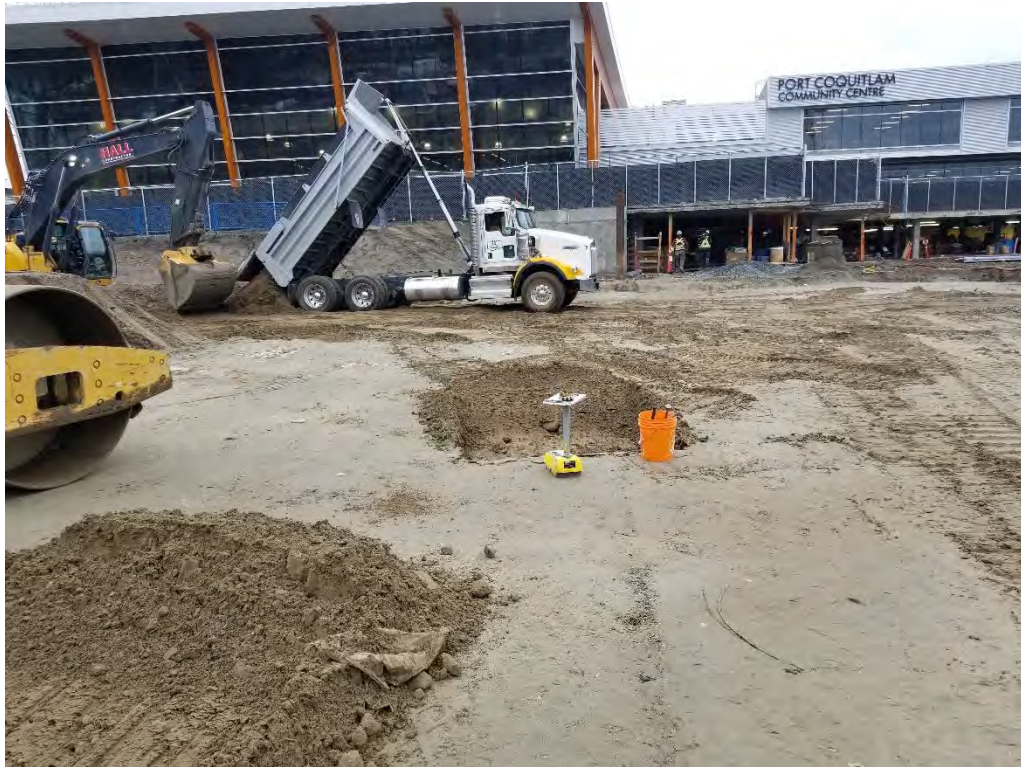
Photo 5 – Fill placement for the access ramp (Item 5). [photo taken by JAL and dated 20191118]
