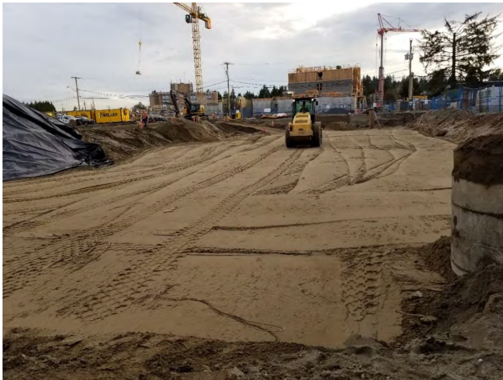
Photo 6 – Recompacting of third lift for the second time. [photo taken by JAL and dated 20191114]
