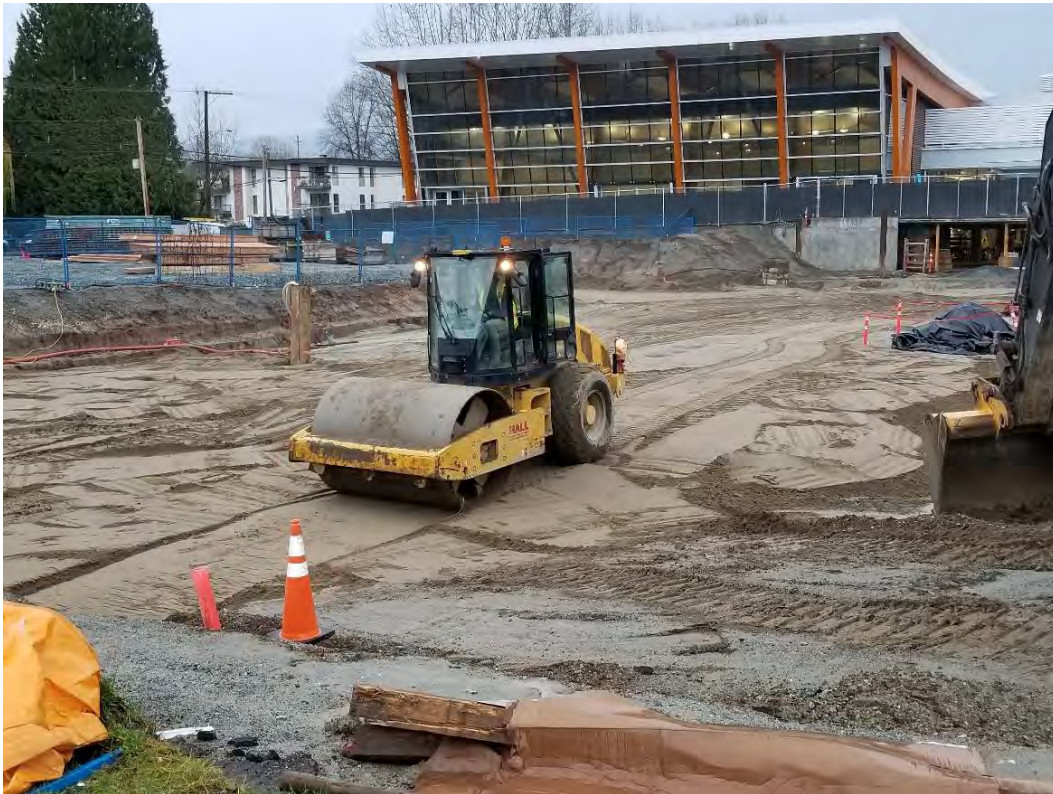
Photo 4 – Compaction of river sand fill at south end of excavation (Item 4). [photo taken by JAL and dated 20191118]
