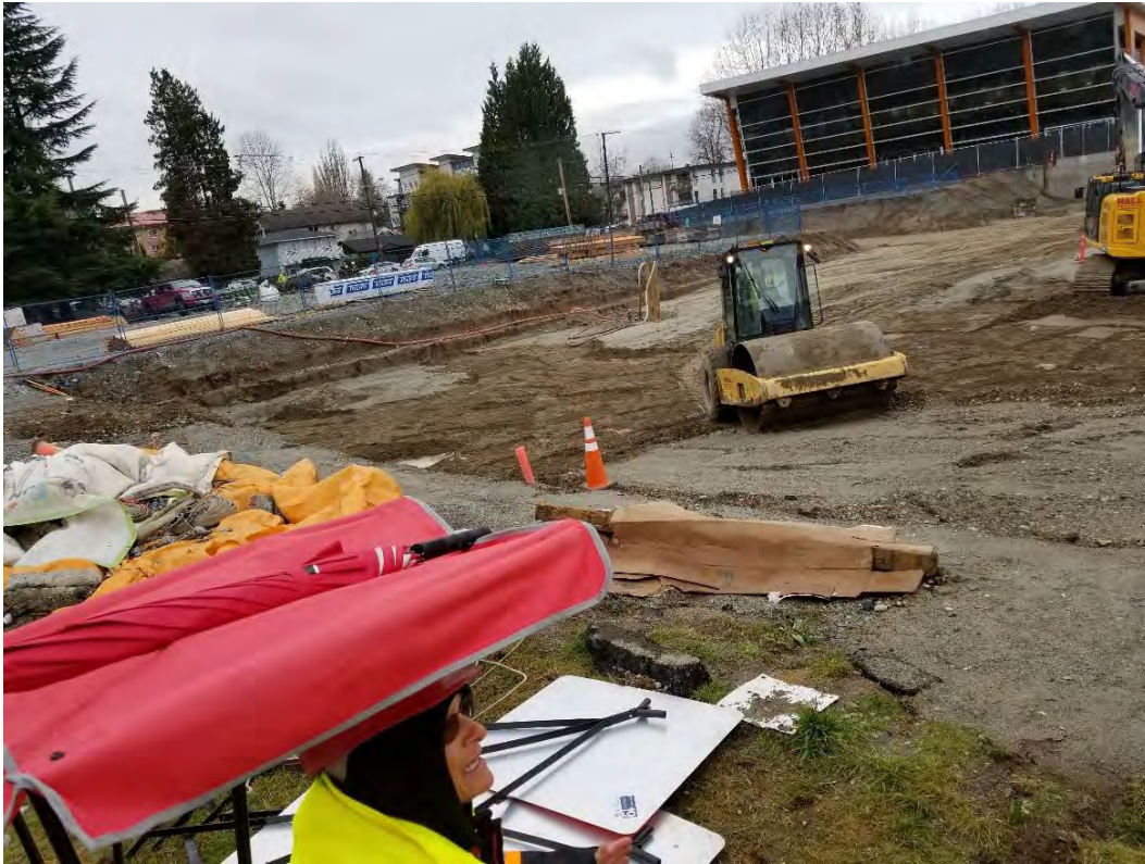
Photo 3 – Compaction of the disturbed surface prior to fill placement (Item 4). [photo taken by JAL and dated 20191118]
