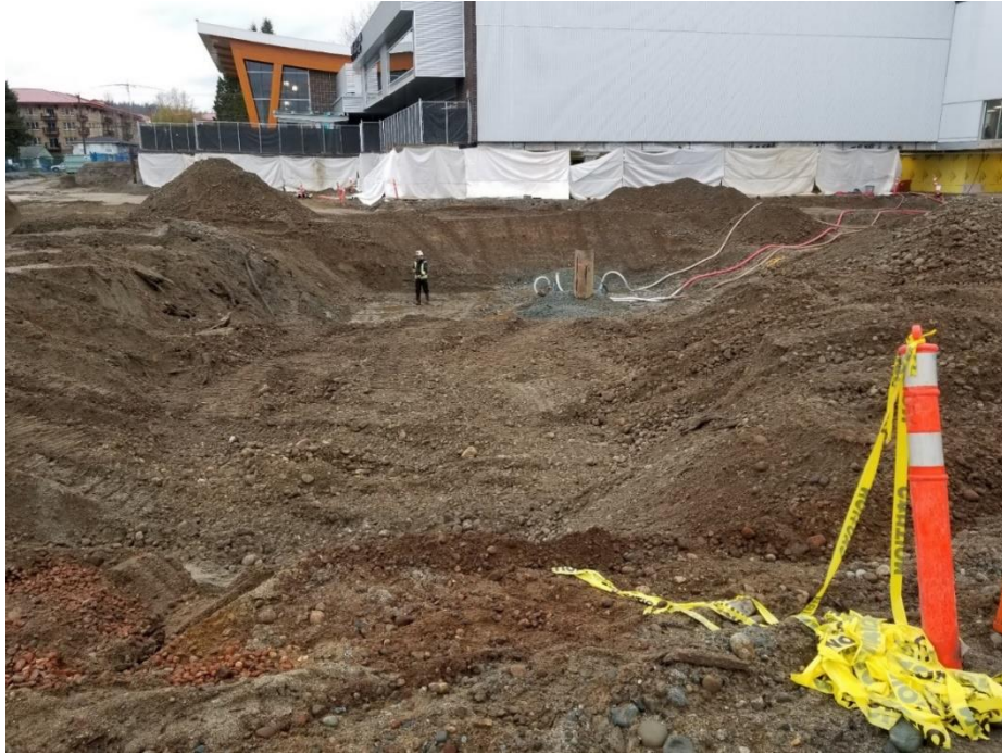
Photo 1 – Looking west. During subgrade approval of the new excavation in the north parkade area (Item 2). [photo taken by JAL and dated 20191203]
