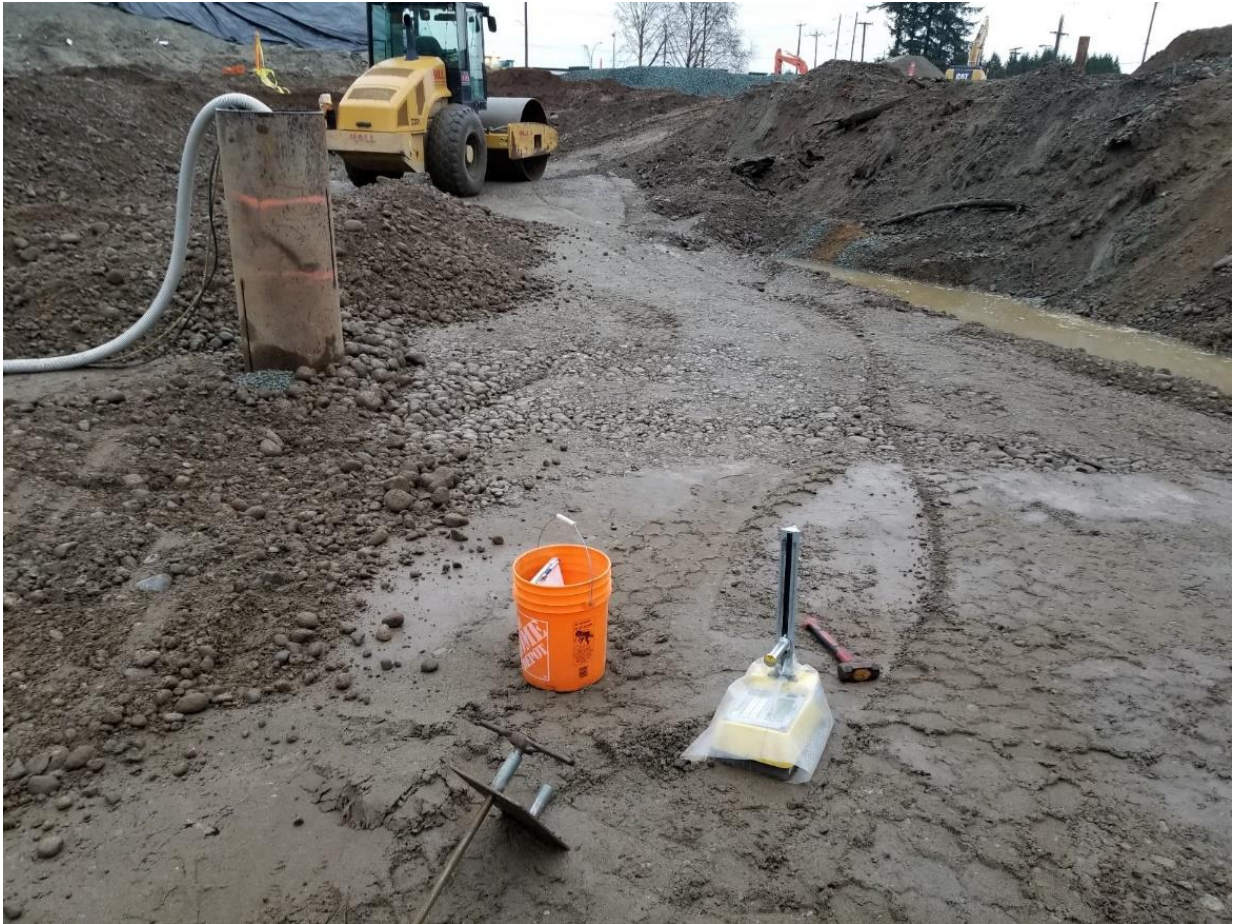
Photo 3 – Looking southeast. During compaction testing of 1st lift (FDR 019-2). [photo taken by JAL and dated 20191203]
