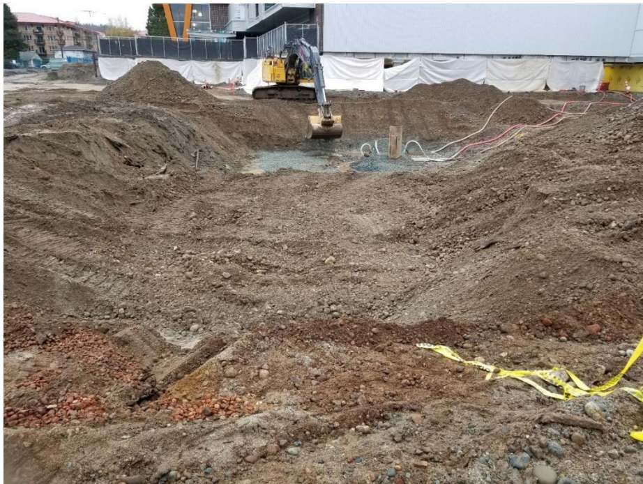
Photo 2 – Looking west. Locally placing 19 mm minus clear crush at the base of the excavation (Item 3). [photo taken by JAL and dated 20191203]
